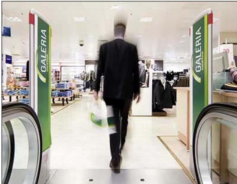
EAS/RFID antennas provide security monitoring at entrances, exits and fitting room areas.
